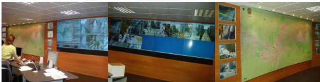
Image 7: Traffic visualization system and control of the traffic with new traffic equipment
